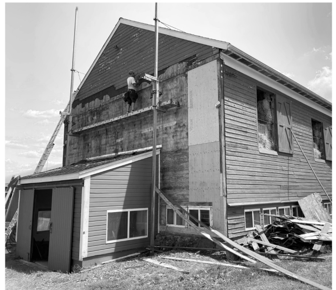
Contractors replacing the siding and sheathing at our Town Line Farm Preserve.
